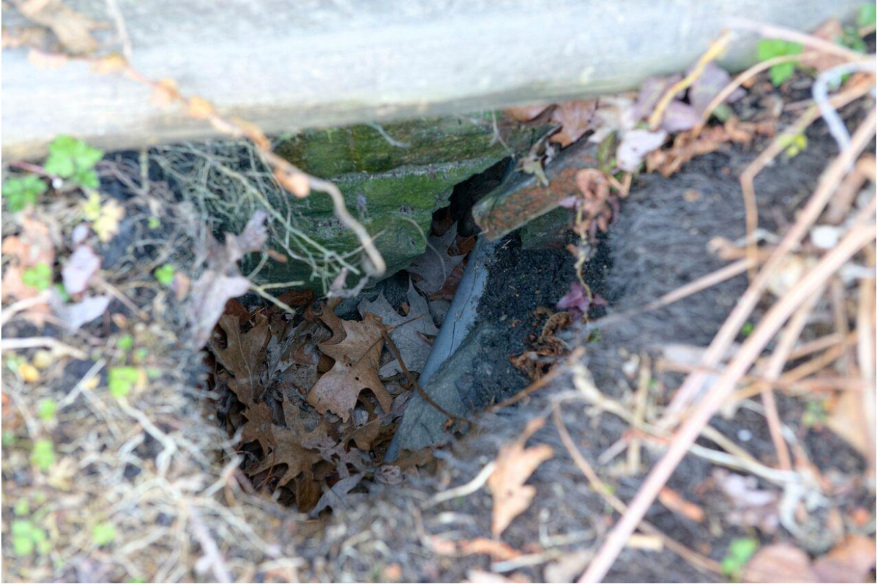
Pictured: Hole on southeast side of building.
