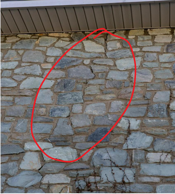
Pictured: Cracks in rear wall.
