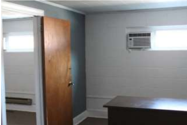
Figure 22: Interior view of 114 W. Swannanoa's 2nd Floor available for rent. The ceiling likely requires asbestos remediation and has evidence of leaks in several places.
